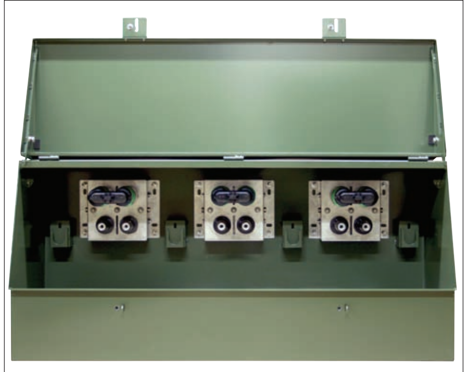
Figure 1. Three-Phase 15 kV Class Clēer SecTER Cabinet.
